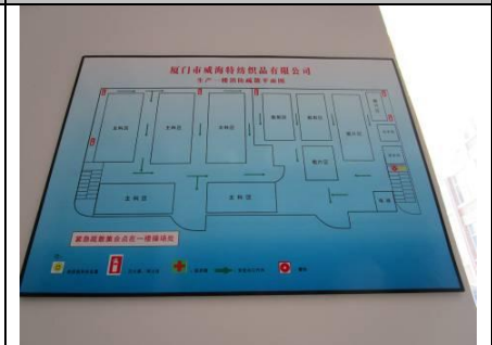
Image 30: The viewer's location was marked wrongly in one fire evacuation plan posted on the 1 st floor of production building.
