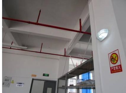
Image 13: Emergency lights and exit signs were installed near or above all fire exits.
