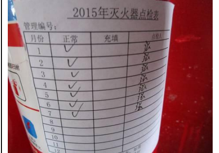
Image 15: Monthly inspection records for fire extinguishers.
