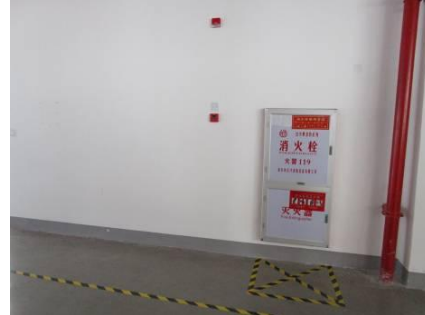
Image 14: Fire alarms and fire fighting equipments were fully installed.
